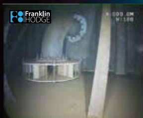
Anti vortex device & suction pipe
