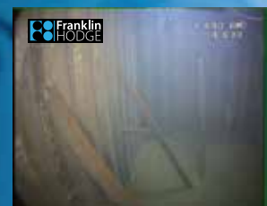
Wall support struts
